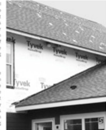
Brackets are in place for the solar domestic hot water and solar electric panels to be installed in the later stages of construction.
